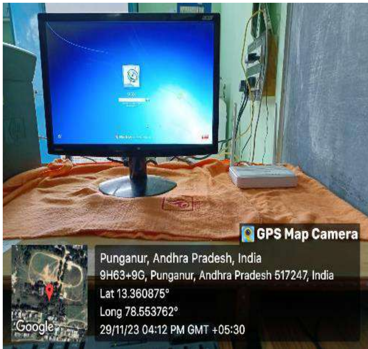
3. BSNL fiber net WIFI Modem in Office room
